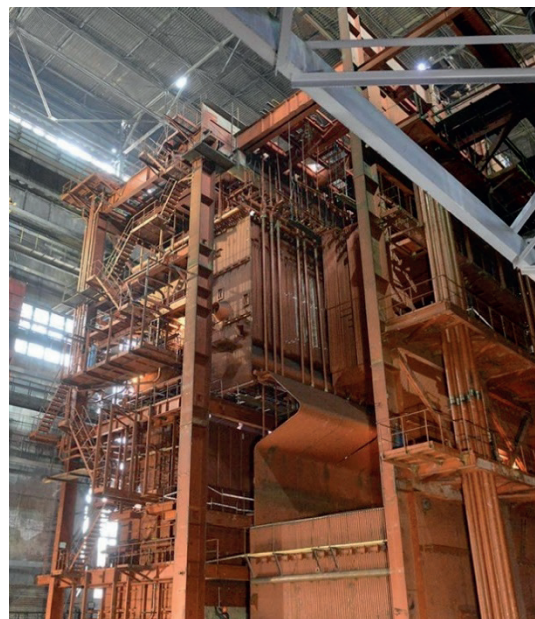
Figure 1. Metal frame with suspended equipment (steam boiler)
