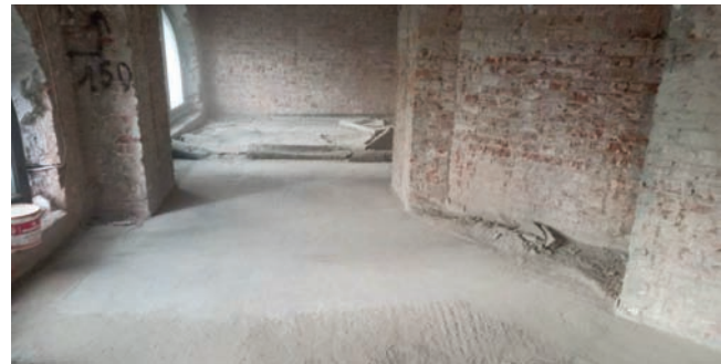
Figure 9. The appearance of structures of the History Museum building before the reinforcement
