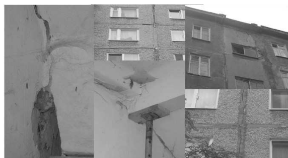
Fig. 2. The panel building structural failure.
