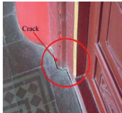
Figure 1. The Xi'an Bell Tower foundation cracking due to periodic forced vibrations caused by underground railway transport
