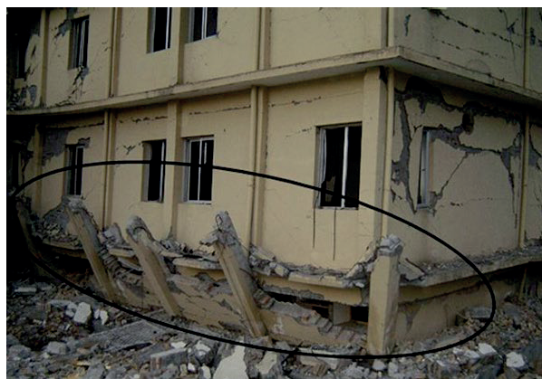
Figure 1. Soft first story collapses during Boumerdes Earthquake, Algeria 2003. [1-4]
