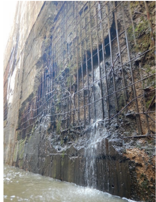
Figure 2. View of the right wall of section No.1 with a sloping crack extending to the face, with voids, exposed reinforcement and water leaks (before overhaul)
