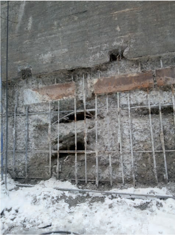
Figure 4. View of a wall with sloping cracks extending to the face, with voids, exposed reinforcement and water leaks (before overhaul)
