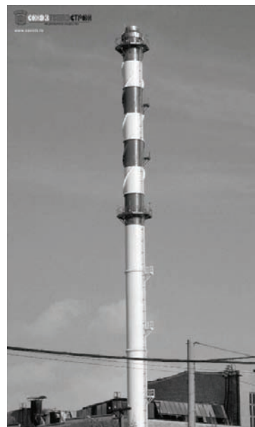
(c) chimney with interceptors
