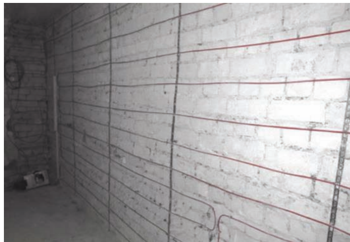
Figure 6. Heating cable on the inner surface of the wall of one of the living rooms of the dormitory.
