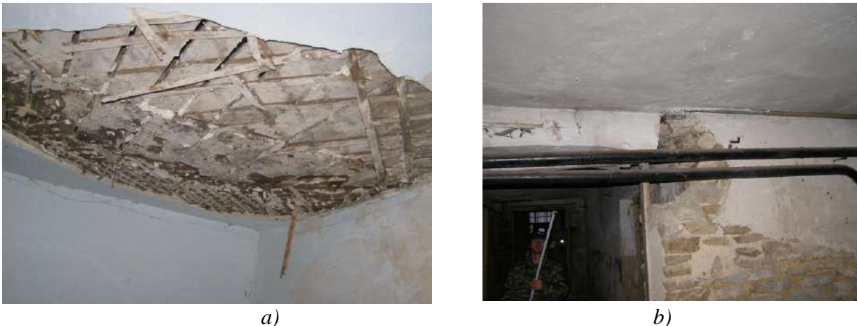
Figure 8. Defects detected during evaluation of technical condition of the building structures: a) floor slabs got wet; b) load-bearing wall in the basement of the building is destroyed.
