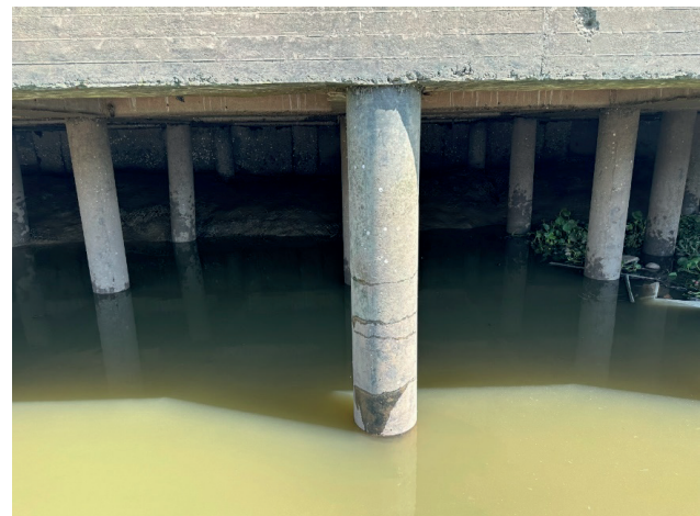
Figure 4. Cracks on piles
