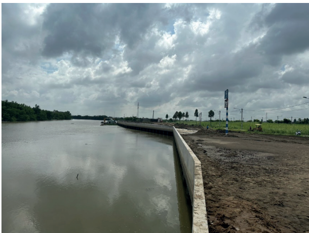
Figure 3. Settlement of the compacted sand layer after construction completion
